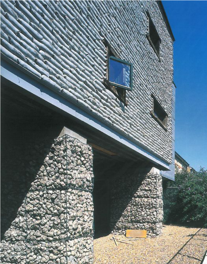
Sandbag wall at Stock Orchard Street Studios, N London by Sarah Wigglesworth Architects
